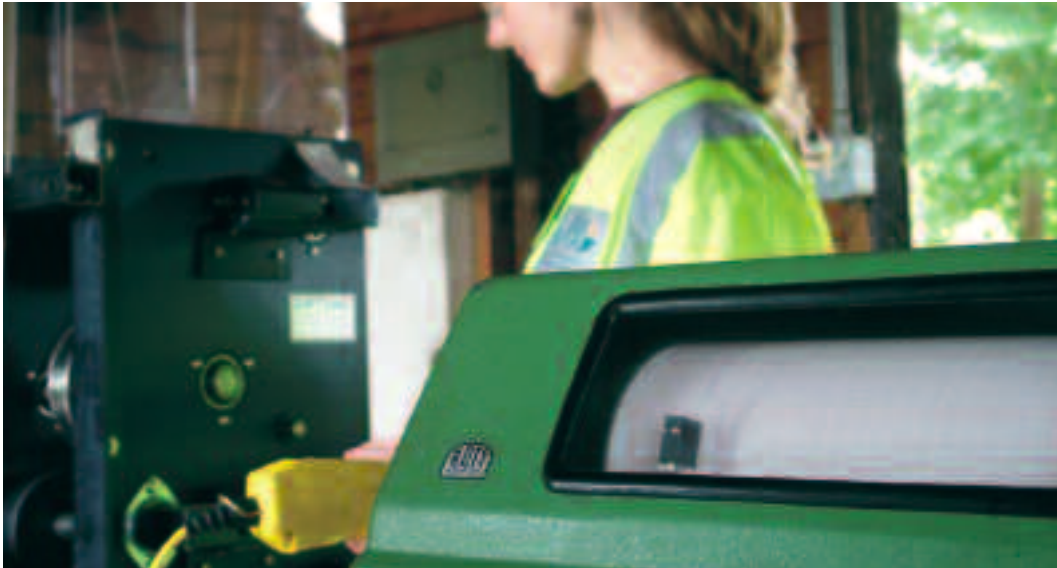
River level monitoring equipment
